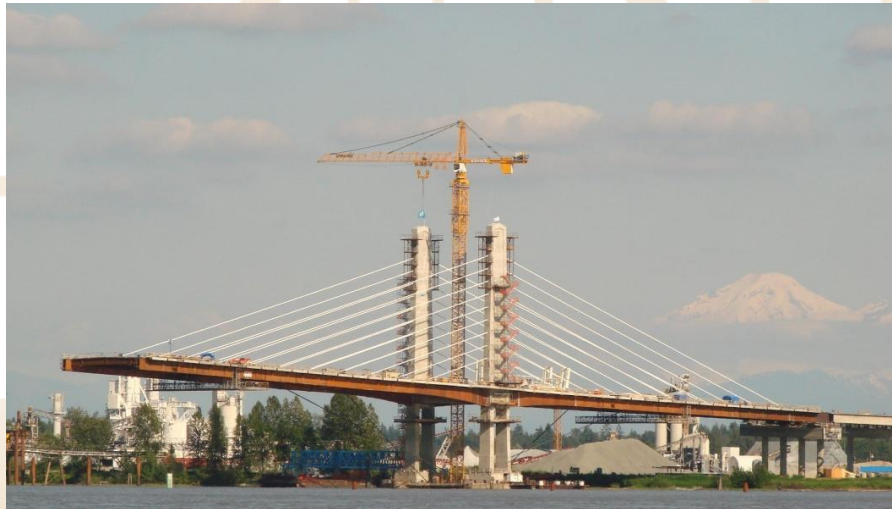
2008 Golden Ears Bridge, Vancouver, BC. “Pile pad” on floating piles in marine clay.
