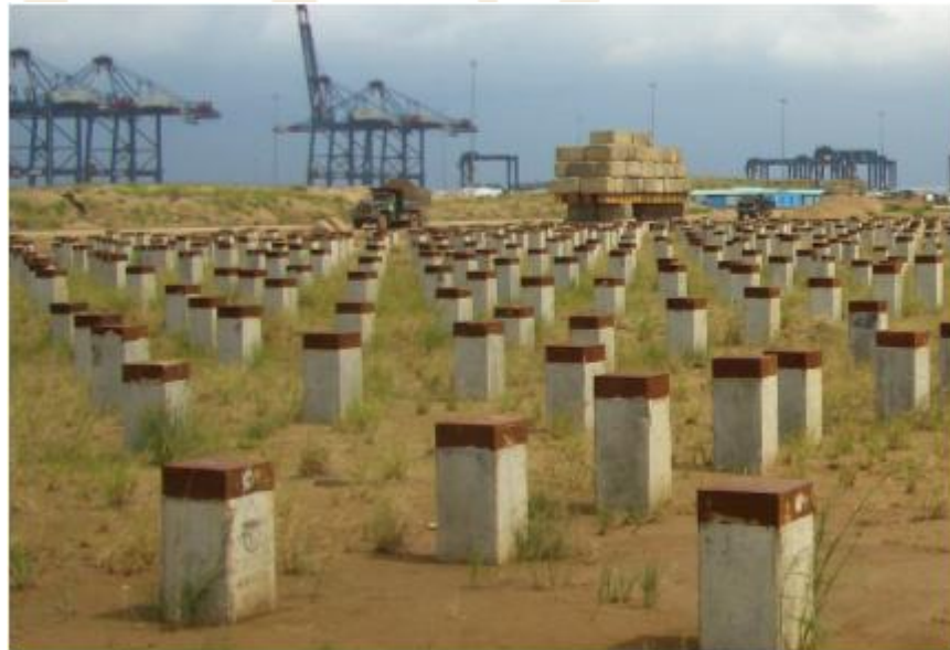
2011 Cai Mep Container Port, Vietnam. Remediation of excessive settlement after a failed wick drain treatment.
