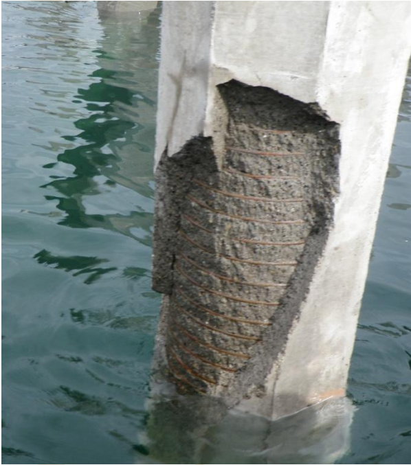
Too thick cover on hard driven piles
